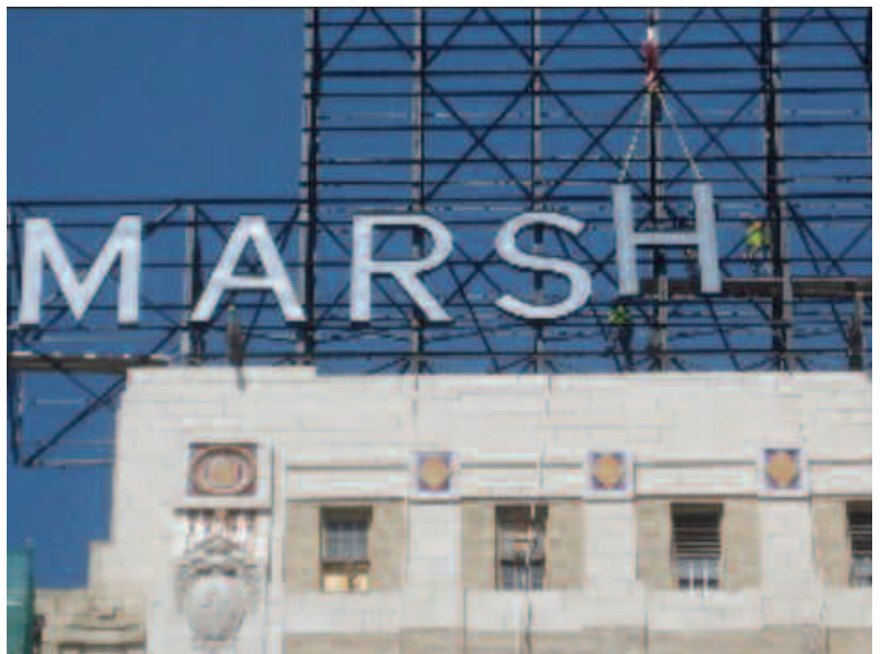
Workers secured an H on the old Hotel John Marshall sign today after it was lifted to the top of the 16-story building by crane.
